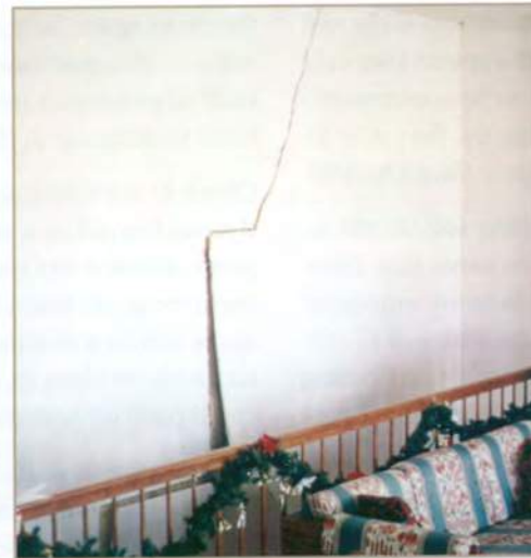
Diagonal cracks in drywall in an interior wall, caused by soil heaving or settling.
