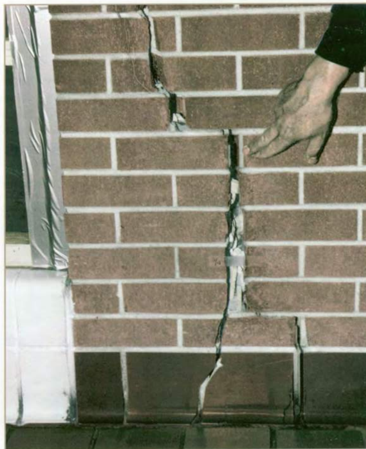
Split bricks and damaged window framing (on left). From Jochim (1987).
