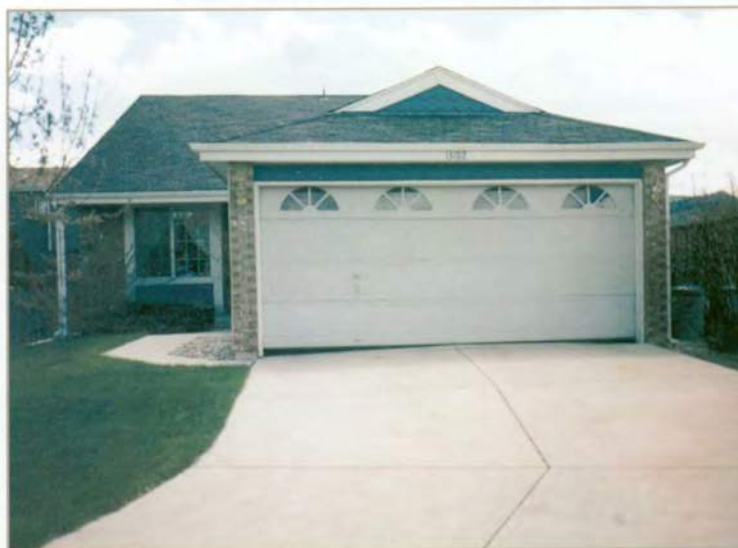
Swelling soil has caused this garage slab to heave and bow at its center. Note the gaps or "batwings" on both sides, where the garage door is not in contact with the slab.
