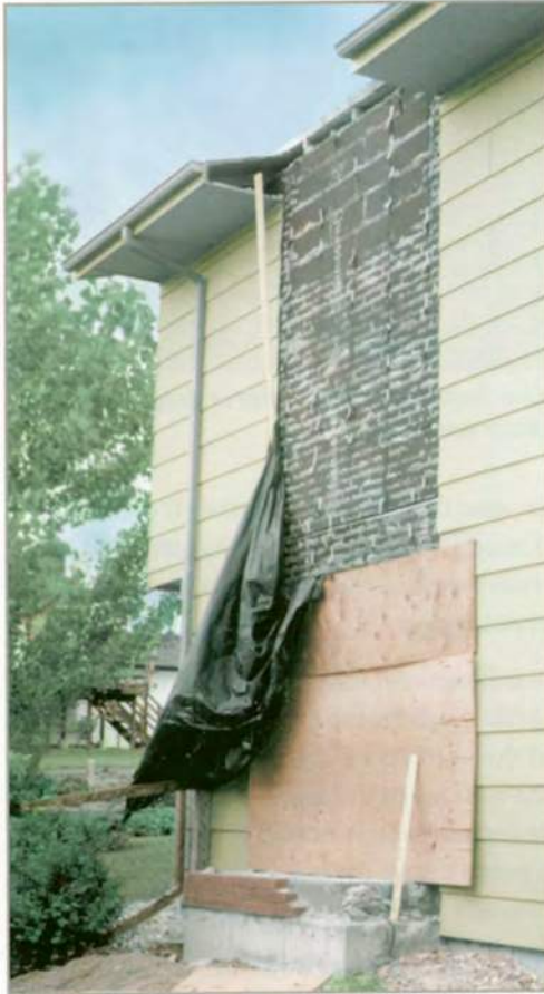
The chimney of this house had separated and tilted away due to swelling soil heaving and had to be removed before it collapsed. From Jochim (1987).
