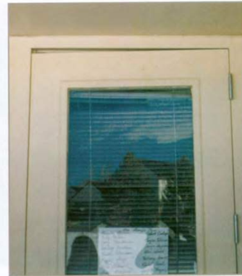
Door frame wedged against the door jamb by heaving of swelling soil. The door binds and does not open or shut easily.
