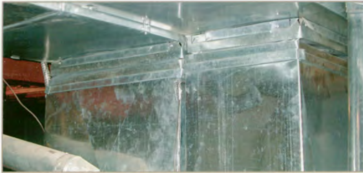
The flexible boot at the top of this furnace has collapsed, leaving it vulnerable to damage if further heaving of the underlying soil and slab floor occurs.
