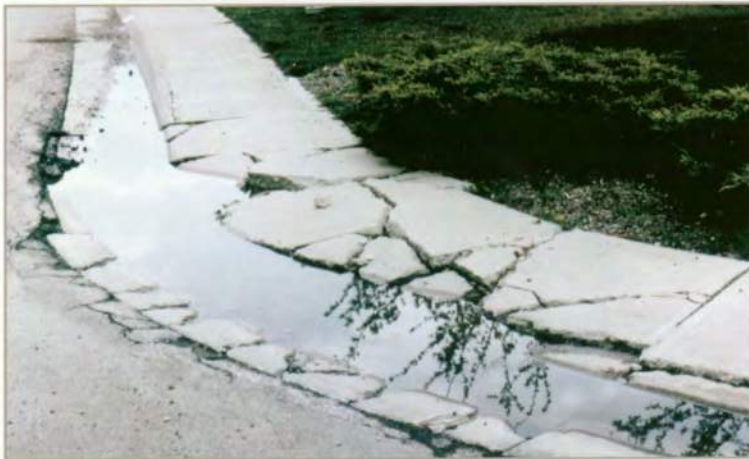
Swelling soil is responsible for the destruction of this sidewalk. Note the ponded water in the street, which could infiltrate through cracks and into the soil.
