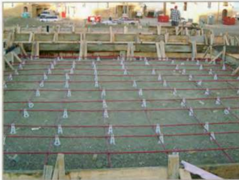
Steel rebar has been placed before pouring concrete for this reinforced slab.
