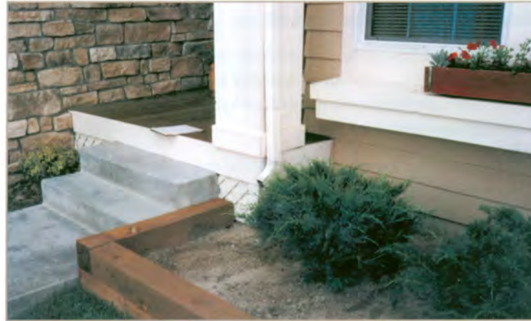
An example of how not to landscape for swelling soil conditions. A garden has been planted next to the foundation, and the downspout extension has been removed.
