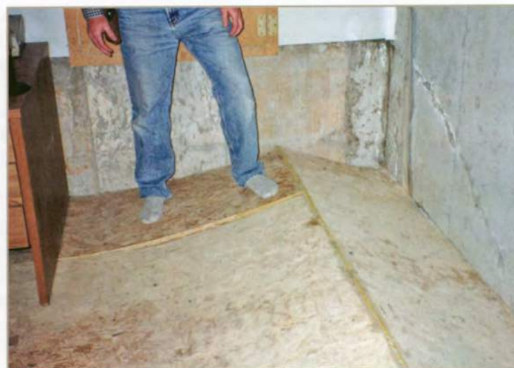
This structural wood basement floor has buckled after undergoing intense heave and lateral pressure from swelling soil.
