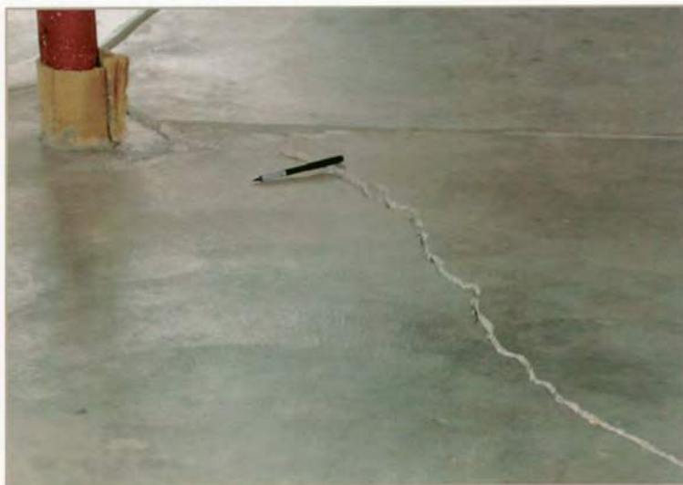
This concrete slab is broken and shows an offset due to differential heaving.
