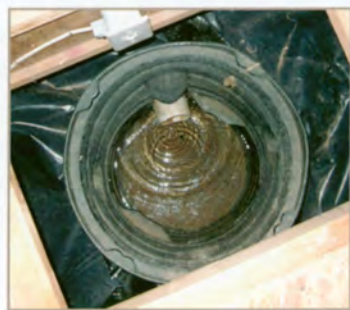
Looking down into a sump pit that has standing water and constant inflow from the two drain pipes.
