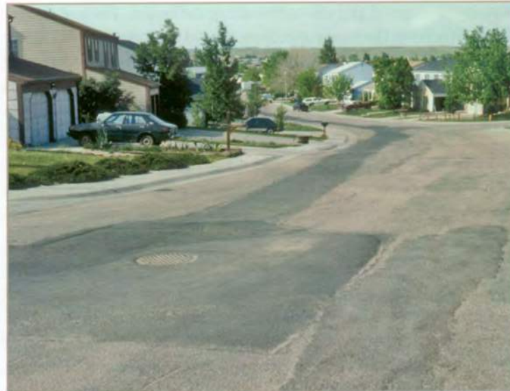
The asphalt patches seen in this street are indicators of multiple repairs and swelling soil.
