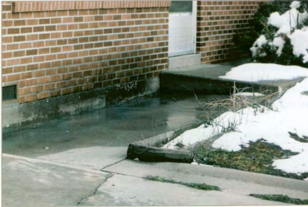
Settling of the backfill material has caused this sidewalk slab to settle and crack, resulting in reverse drainage and ponding next to the foundation. From Jochim (1987).
